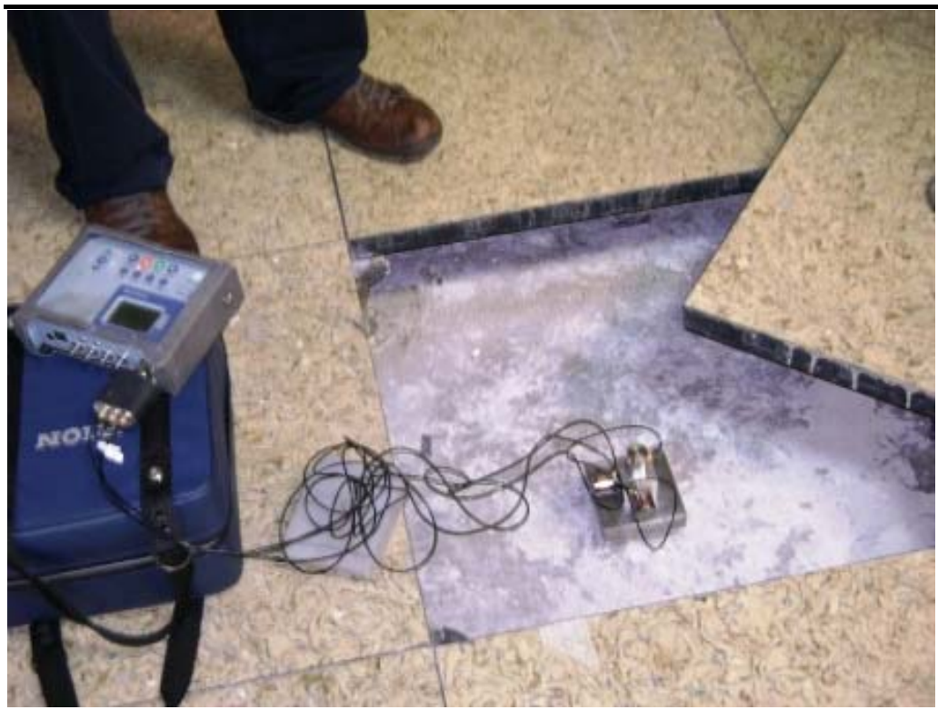
Figure A 1.7 Mater Private: Concrete floor in room adjacent to MRI machine
