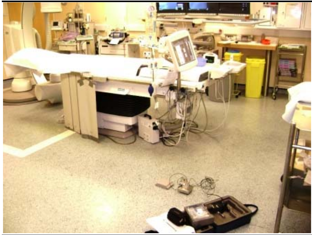
Figure A1.12 Mater Private: Cath Lab 2 – Radioactive Screening and Scanning
